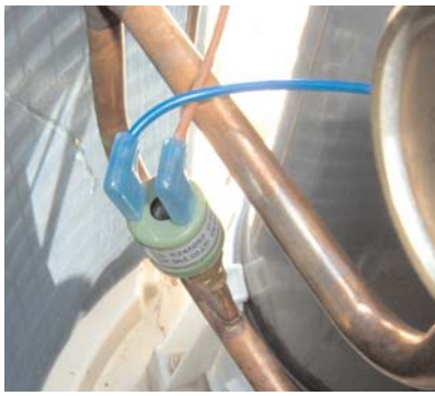
High Pressure Switch (green) open 450 PSi closed 250 PSi
